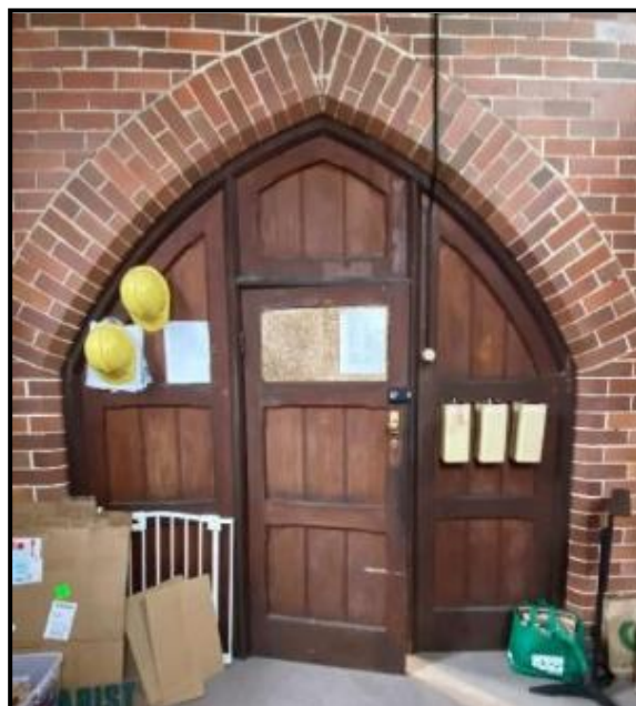
Above: the original solid timber doors now stored over the new ceiling.
